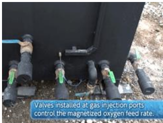
Valves installed at gas injection ports
